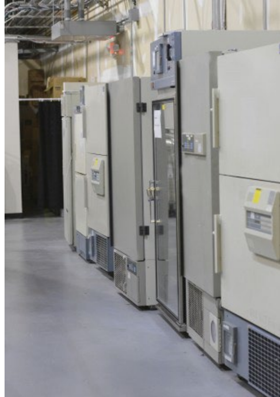
Pharmaceutical warehouse - refrigerated storage 医薬品倉庫-冷蔵保管庫
